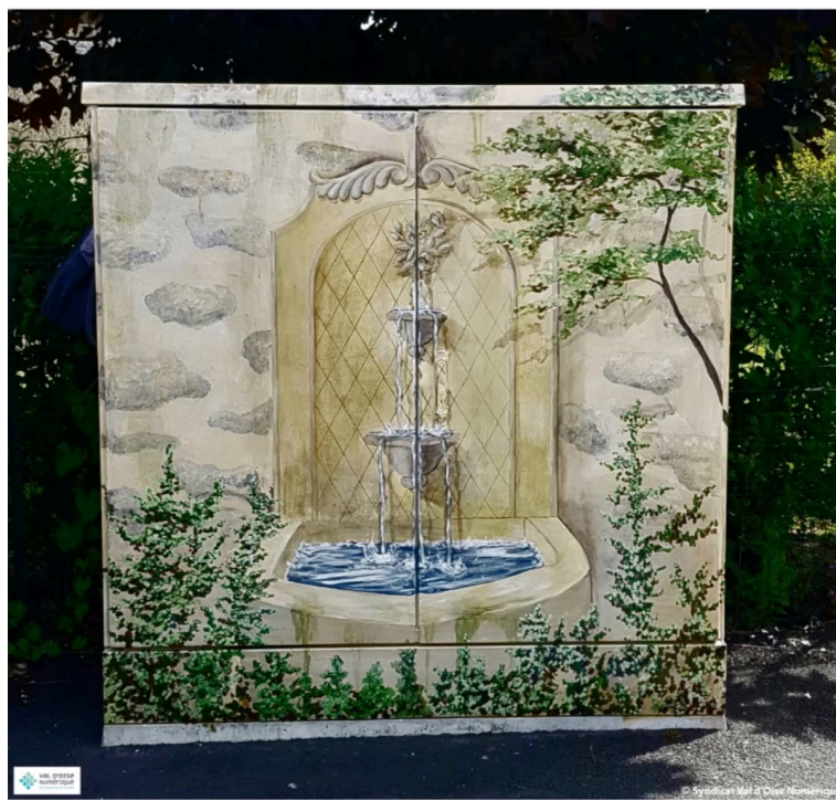
Example of a cabinet from Val d'Oise
